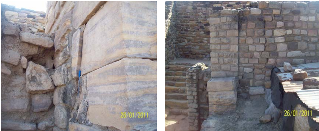
Figure 6: widening of cracks on the wall of north gate.
